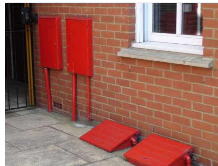
Avoid visual clutter from building services and service boxes
